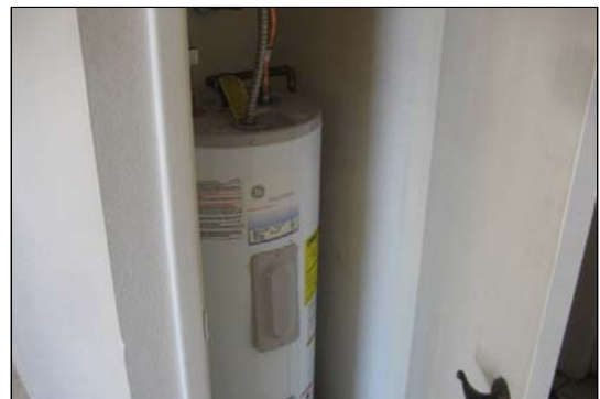
Apt No. 15 – Two-bedroom apartment with hot water heater in easy-access hall closet
