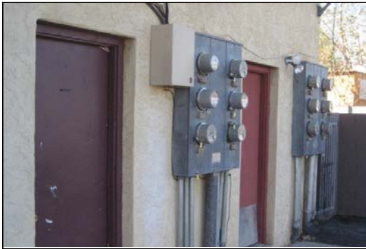
Individually metered for electricity
