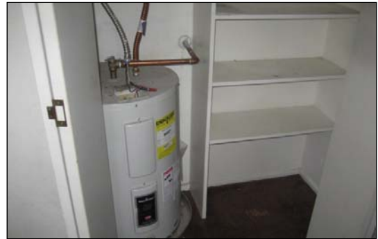
Apt No. 3 – Large two-bedroom showing hot water heater in easy-access pantry
